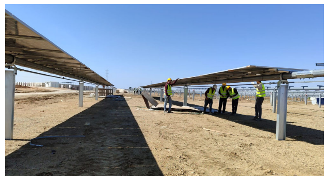
100 MW Kairouan Photovoltaics Plant, Tunesia, 2023 – 2025
